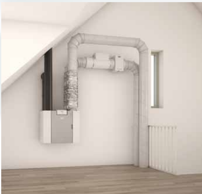
The Pure induct is installed directly downstream of the ventilation appliance.
